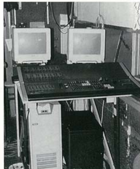
Main Console, UPS (white box) and LP90 Electronics Tower (black box) underneath.
